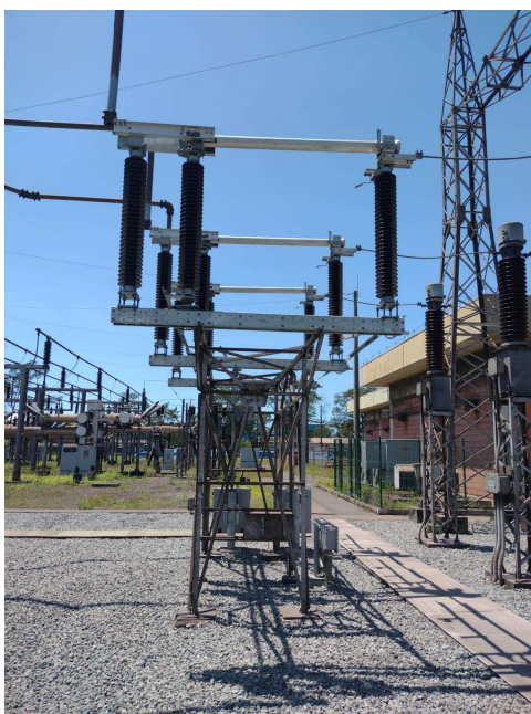
Figure 2. Vertical Disconnect Switch
