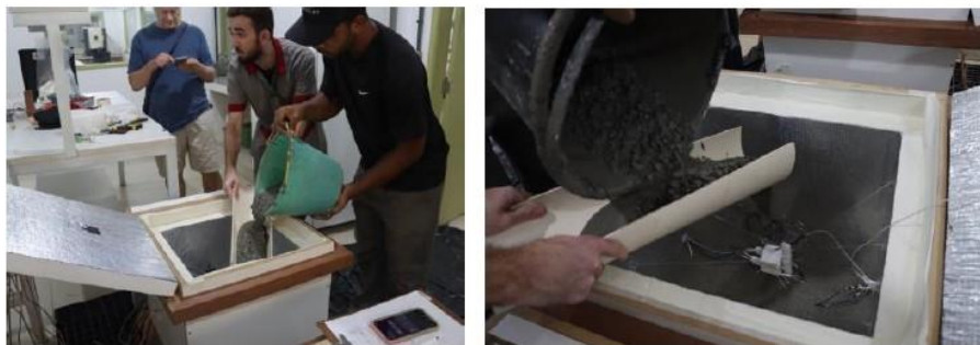
Figure 1. Block concreting being carried out at the LABEST/NUMATS laboratory (Toledo Filho et al. [2])
