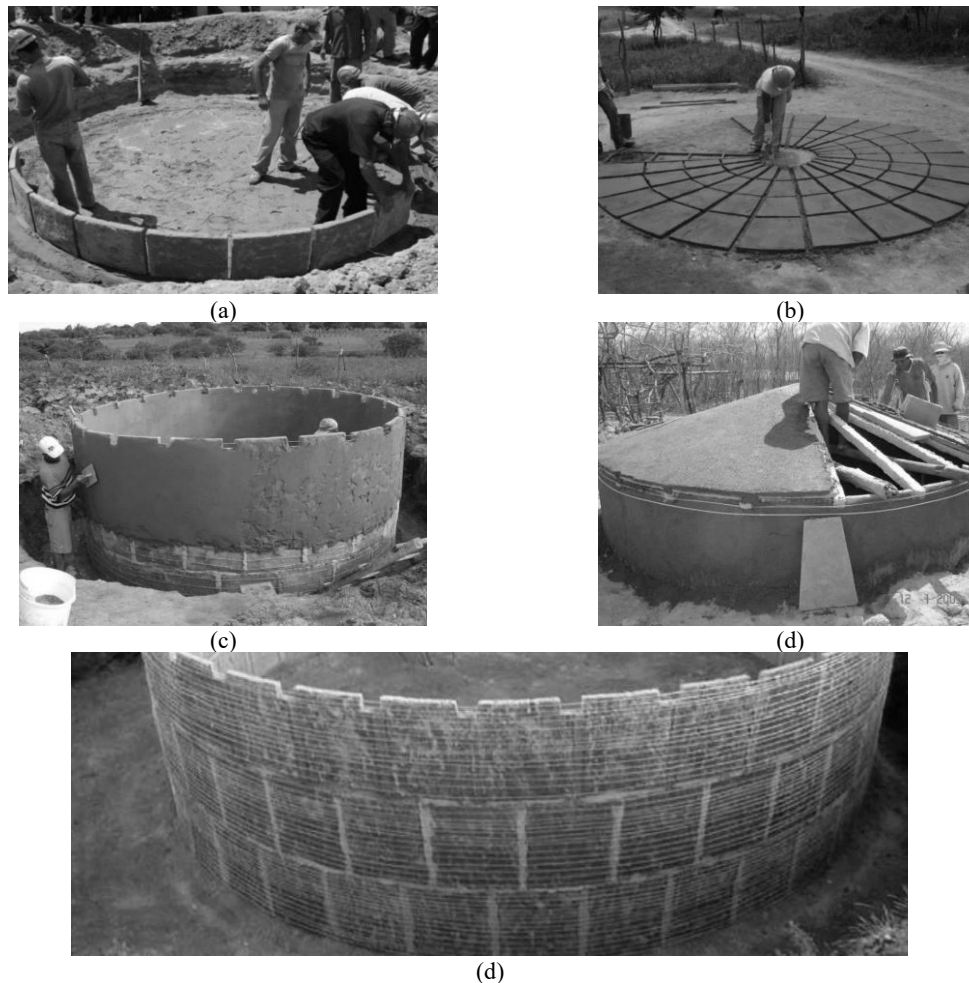
Figure 1 - a) Positioning of the first row of plates; (b) Casting of the plates; (c) Coating of the walls; (d) Execution of the walls; (e) Detail of the arrangement of steel wires (ASA [6])
