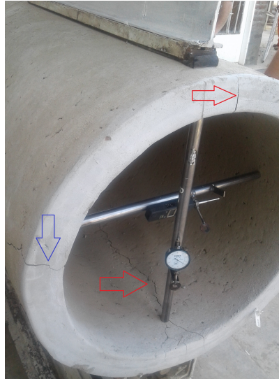
Figure 12. Flexural cracks in a pipe subjected to the TEBT.
