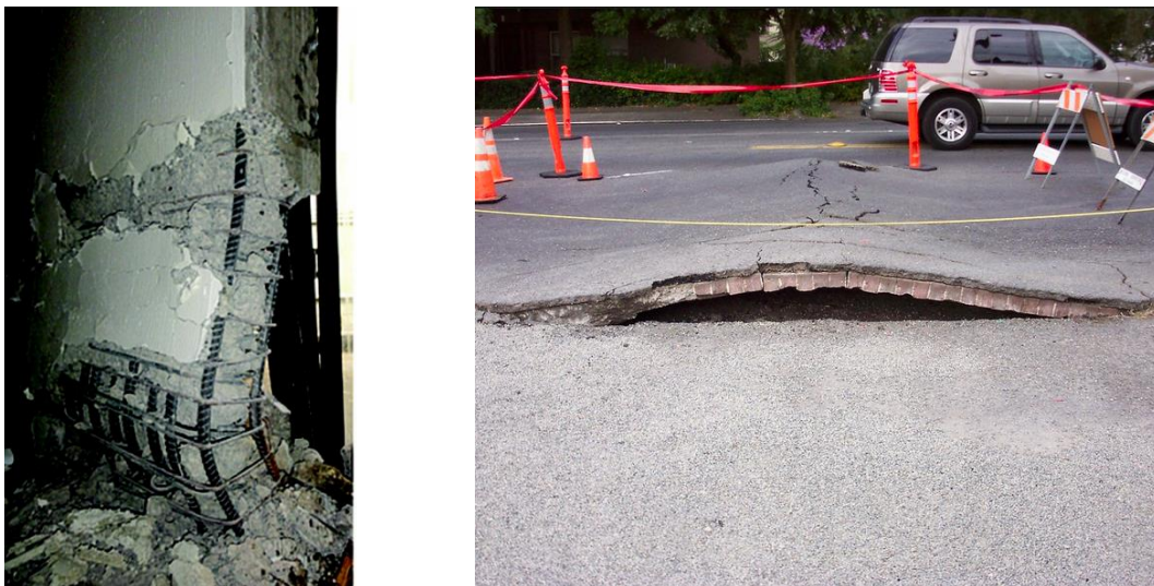
Figure 1. a – Rupture and spalling of V-shaped RC shear wall (extracted from [1]). b- Road pavement “blow-up buckling” due to thermal expansion effect.
