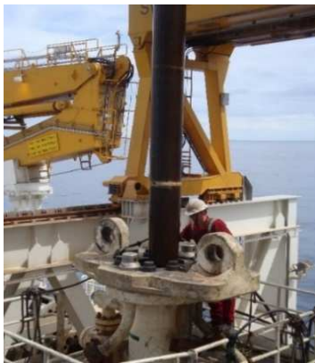
Figure 4 - Pipe cut in BOP commissioning test. Source: Petrobras.
