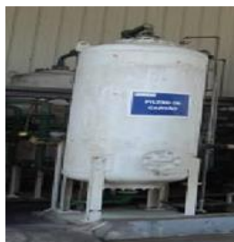
Figure 1 - Photograph of the studied activated carbon filter.
