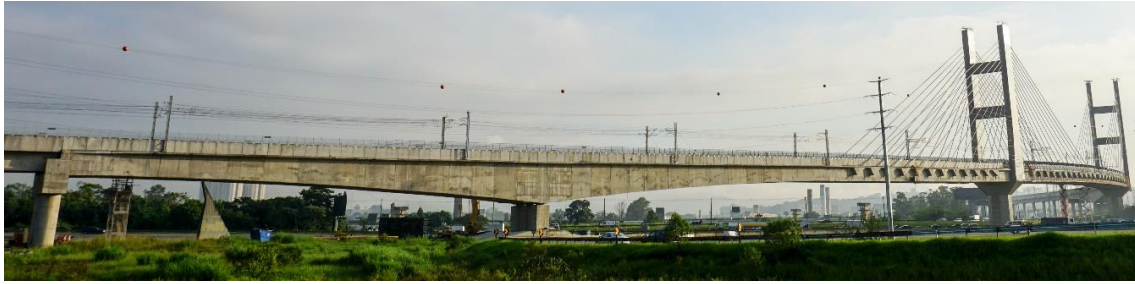
Figure 3. Cable-stayed railway bridge over the Ayrton Senna and Hélio Smidt freeways (Oyamada et al. [14]).
