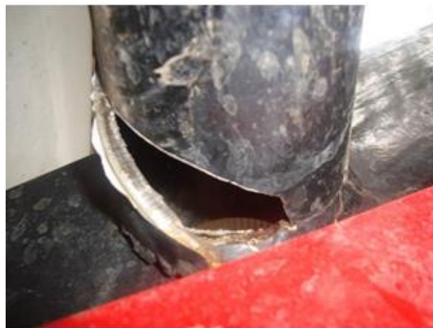
Figure 2 – The failure in the weld area
