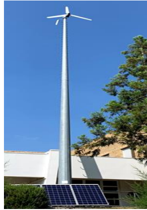
Figure 1 - Small wind turbine tower, Bragança - Portugal
