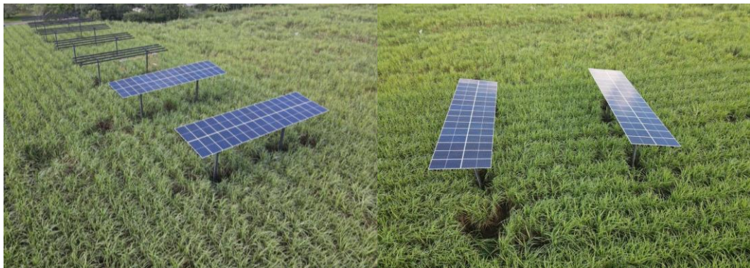
Figure 3. Overview of the structural unit supporting the photovoltaic solar panels.
