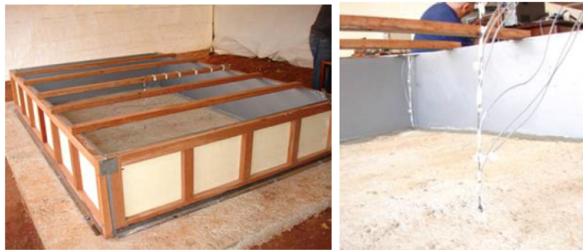
Figure 5. Slab shape tested and monitoring thermometers coupled to the LYNX platform (COPPE/FURNAS).
