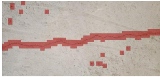
Figure 8. False positives due to stains
