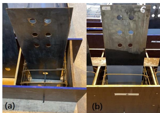
Figure 5 – (a) Model setup without grease and ink before concreting. (b) Model setup with grease and ink before concreting.
